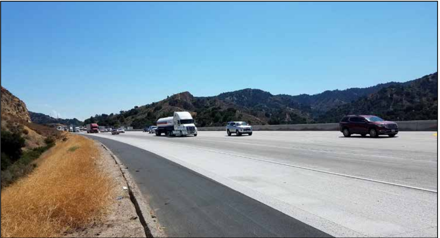
The repaved stretch of Interstate 5 includes the lanes extending from the Newhall Pass toward Calgrove Boulevard. Photo: M. Comeaux for Caltrans
